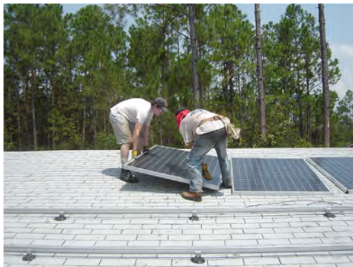
Roof mounted PV, ecoMOD2
