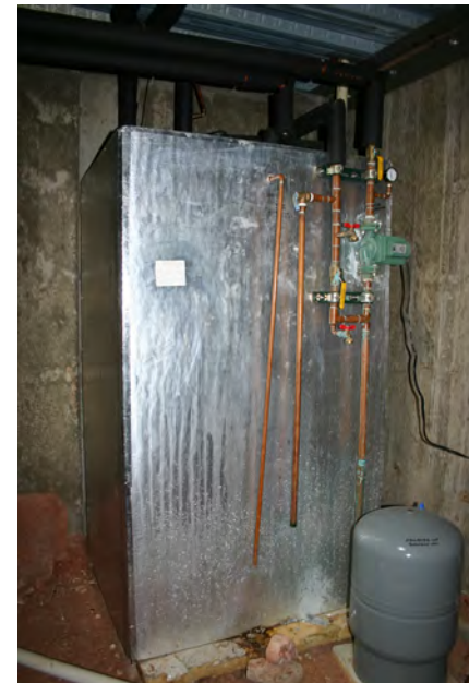
Solar Hot Water Storage Tank, Wild Sage Mechanical Closet Basement
